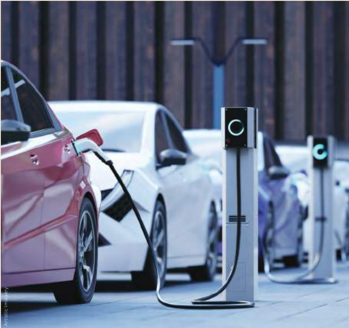
EV Charging Stations
